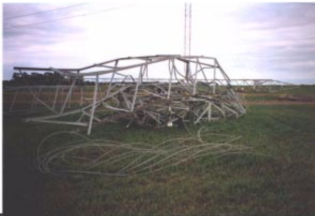
Fig. 1 Damaged HVDC Tower
